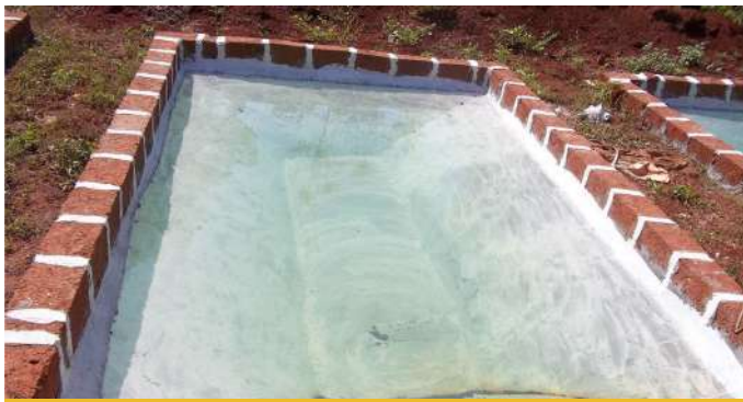
Water Storage Tanks Using Natural Fibers (Image Credit: RuTAG)
