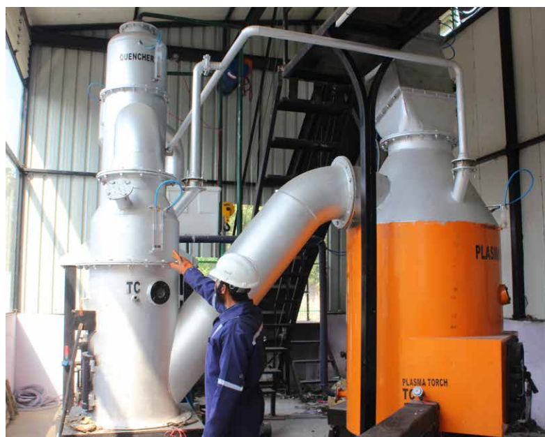
Pilot Installation of Plasma Pyrolysis Unit at Waste to Wealth Technology Park
